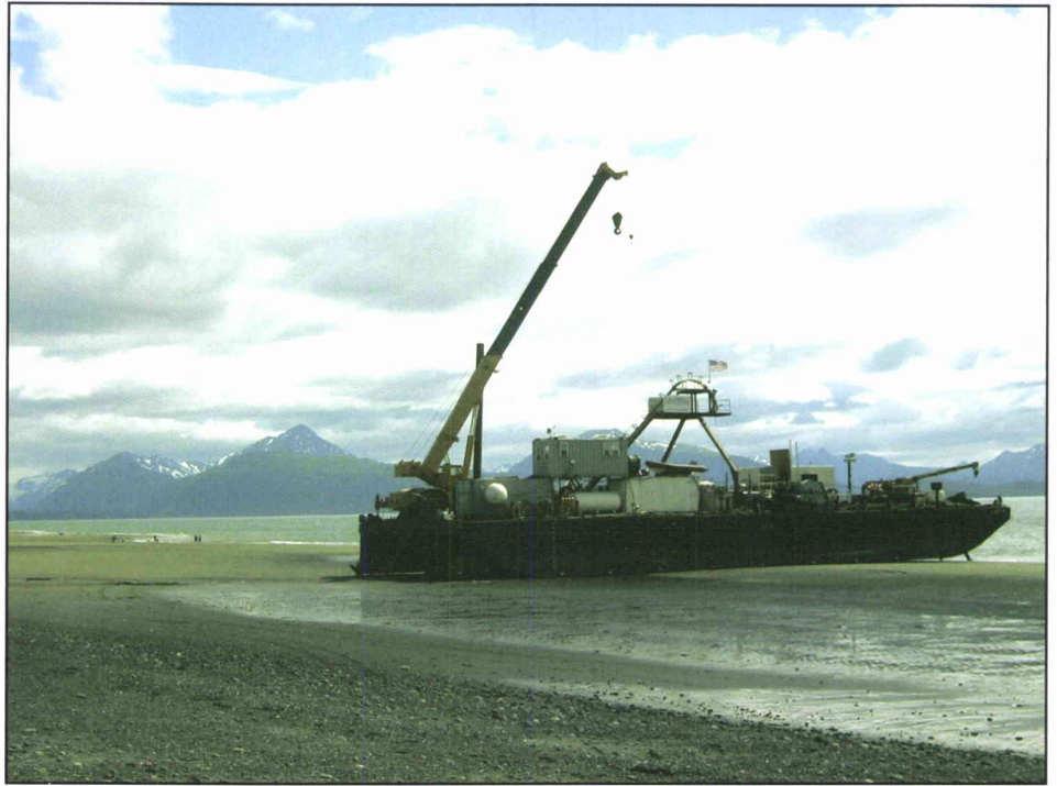
This shallow draft deck barge was utilized by Caldwell Marine for landing the fiber cable at several locations in Alaska.
